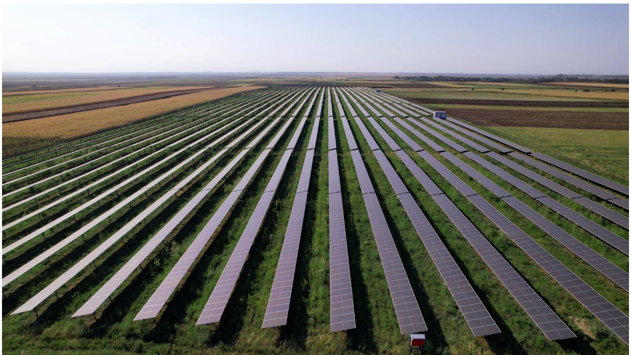
7,1 MWp solar PV power plant Săhăteni | Image source: Photon Energy Group
